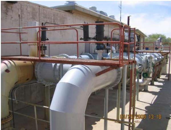
Lift Station #20 Force Main Header
