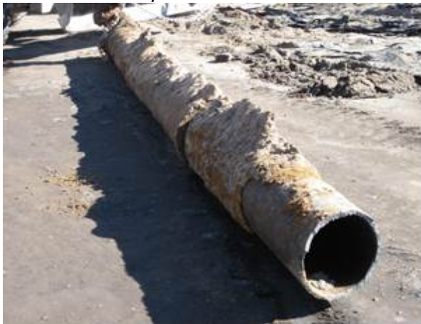
Corroded Steel Pipe
