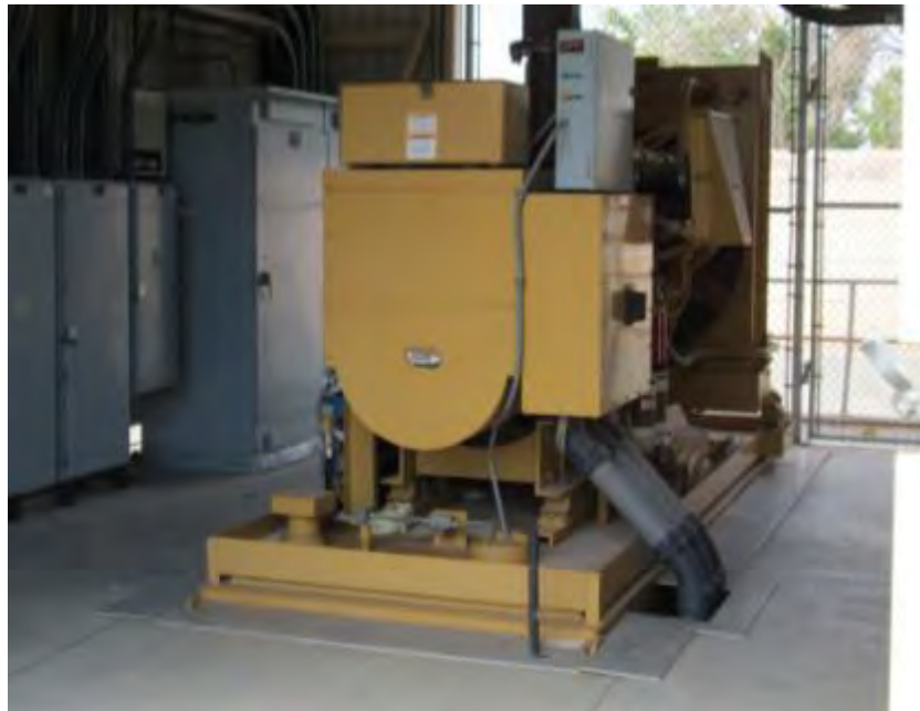
Photograph 2. Pump Station No. 20 – View of backup generator. Authority staff stated that the pump station also has two separate electrical feeds from the local utility, Public Service Company of New Mexico (PNM).
