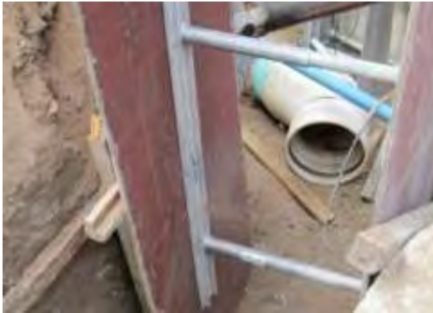
Photograph 15. Mary Ellen Street NE Construction – View of the new 24-inch air jumper line to be connected in the 1200 block of Mary Ellen Street NE.
