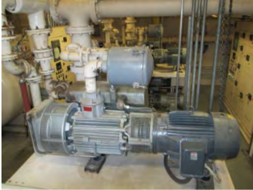
Photograph 5. Vacuum Station Nos. 61 & 64 – View of a vacuum pump inside the building that houses Vacuum Station Nos. 61 & 64.
