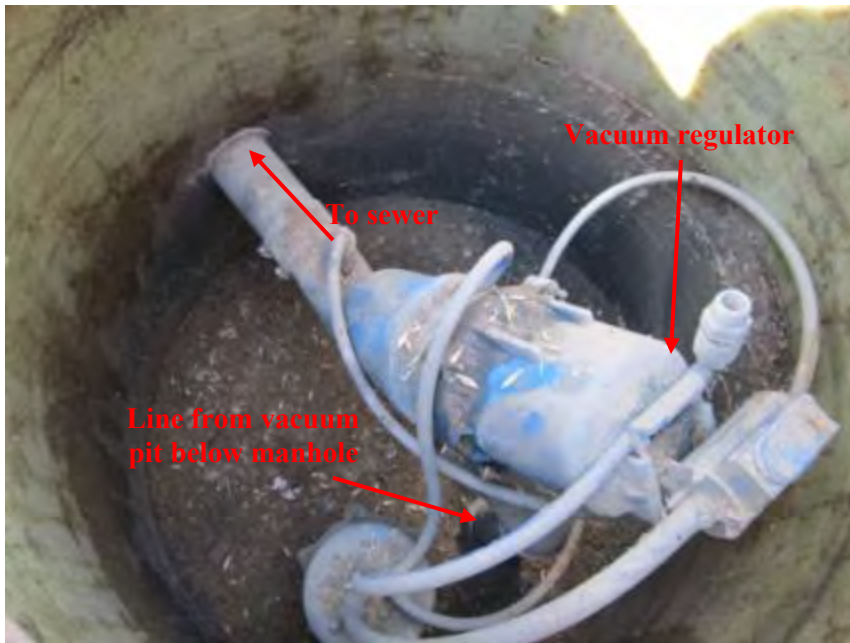
Photograph 6. Vacuum Station Nos. 61 & 64 – View inside a vacuum pit manhole. The regulator turns the pump on when the pit contains approximately 10 gallons.
