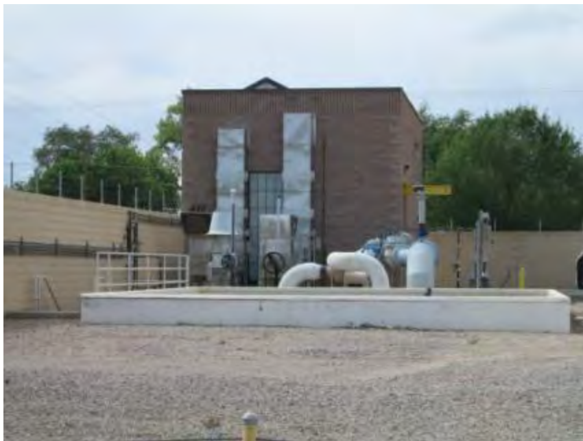
Photograph 4. Pump Station No. 20 – View of the second pump building, which primarily serves as backup capacity, at Pump Station No. 20.
