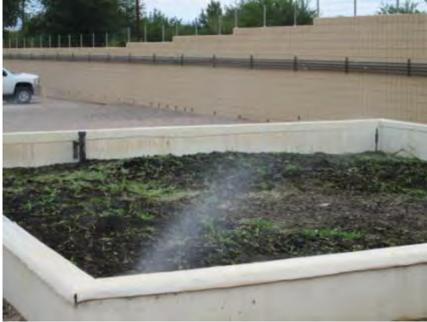
Photograph 3. Pump Station No. 20 – View of the pump station’s biofilter for odor control.
